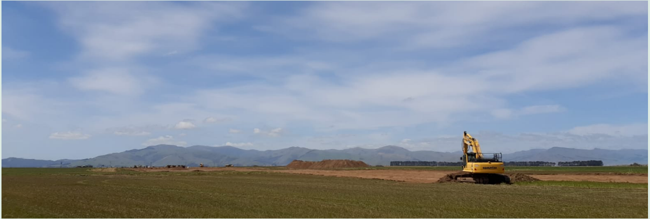
Work starts on upgrading facilities at the Tāwhaki Aerospace Centre at Kaitorete
